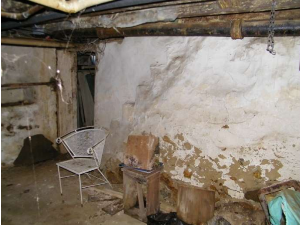
The wall between the basement below the small kitchen and the original basement as viewed from the small kitchen side (note doorway into original basement at left).
